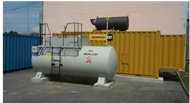
Figure 2. Diesel generator in container design with additional fuel tank
